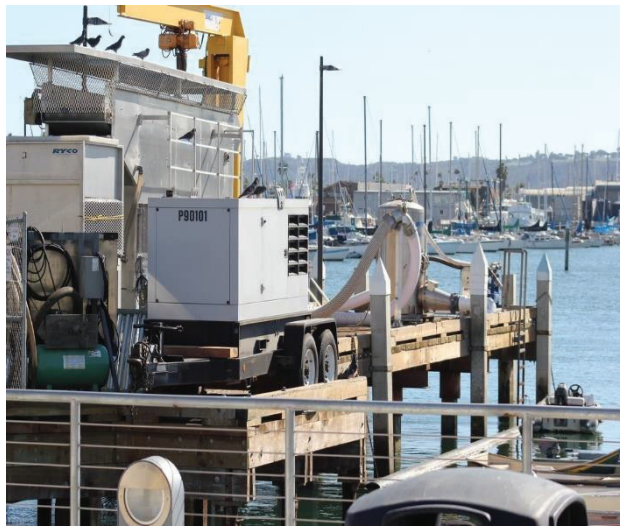
Fig 3.47 - Driscoll’s Wharf Wetfish pump – view from North. Taken September 25, 2017.
