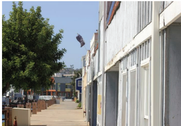
Fig 3.32 – Face of unpainted building at Driscoll's Wharf. Taken October 9, 2017.
