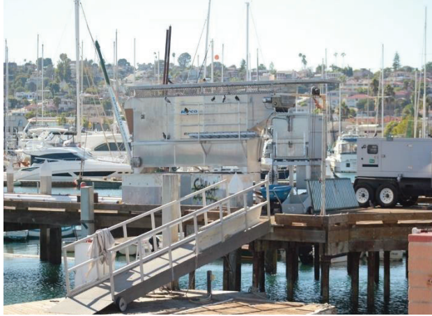
Fig 3.46 – Driscoll’s Wharf Wetfish pump – view from South. Taken September 25, 2017.
