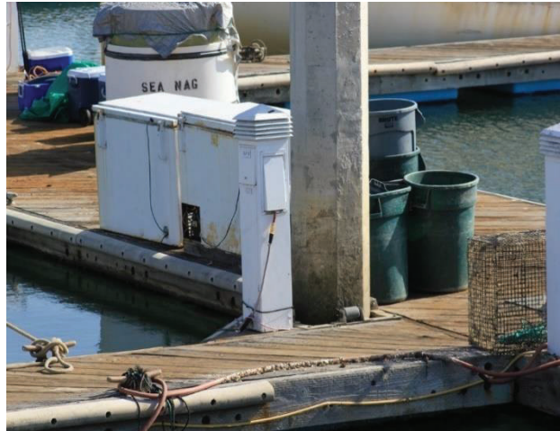
Fig 3.9 – Alternate Shore Power box at Tuna Harbor. Taken October 9, 2017
