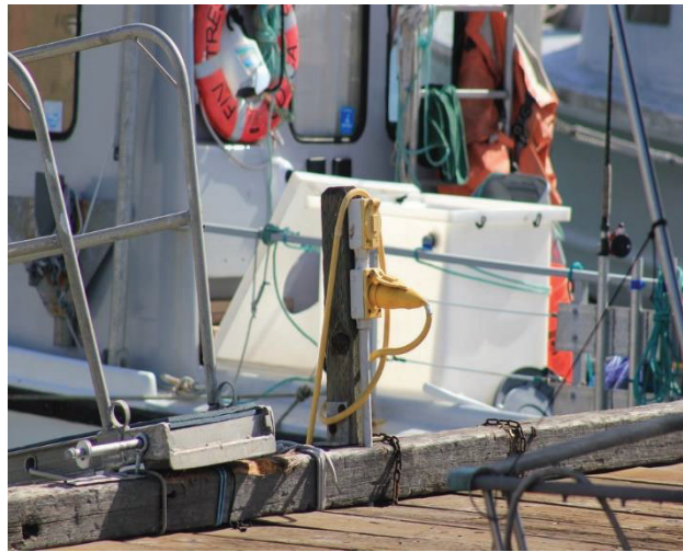
Fig 3.35 - Shore power connections at Driscoll's Wharf. Taken October 9, 2017.
