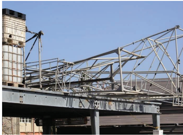
Fig 3.40 - Roof of open structure (stairway leading to rooftop clearly seen in above photo) with swordfish planks. Taken October 9, 2017.
