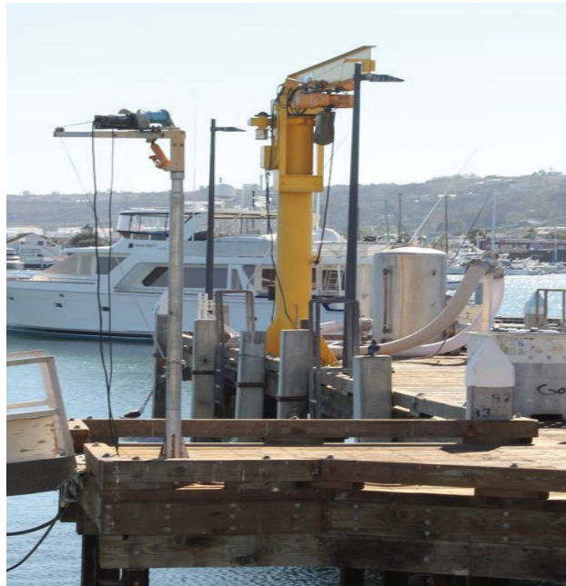
Fig 3.43 - Driscoll's Wharf Offloading Crane – the yellow crane towards the end of the Pier. Taken September 25, 2017.
