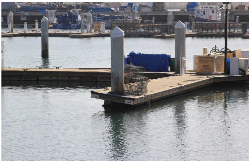
Fig 3.4. Tuna Harbor dock damage. Taken - October 10, 2017
